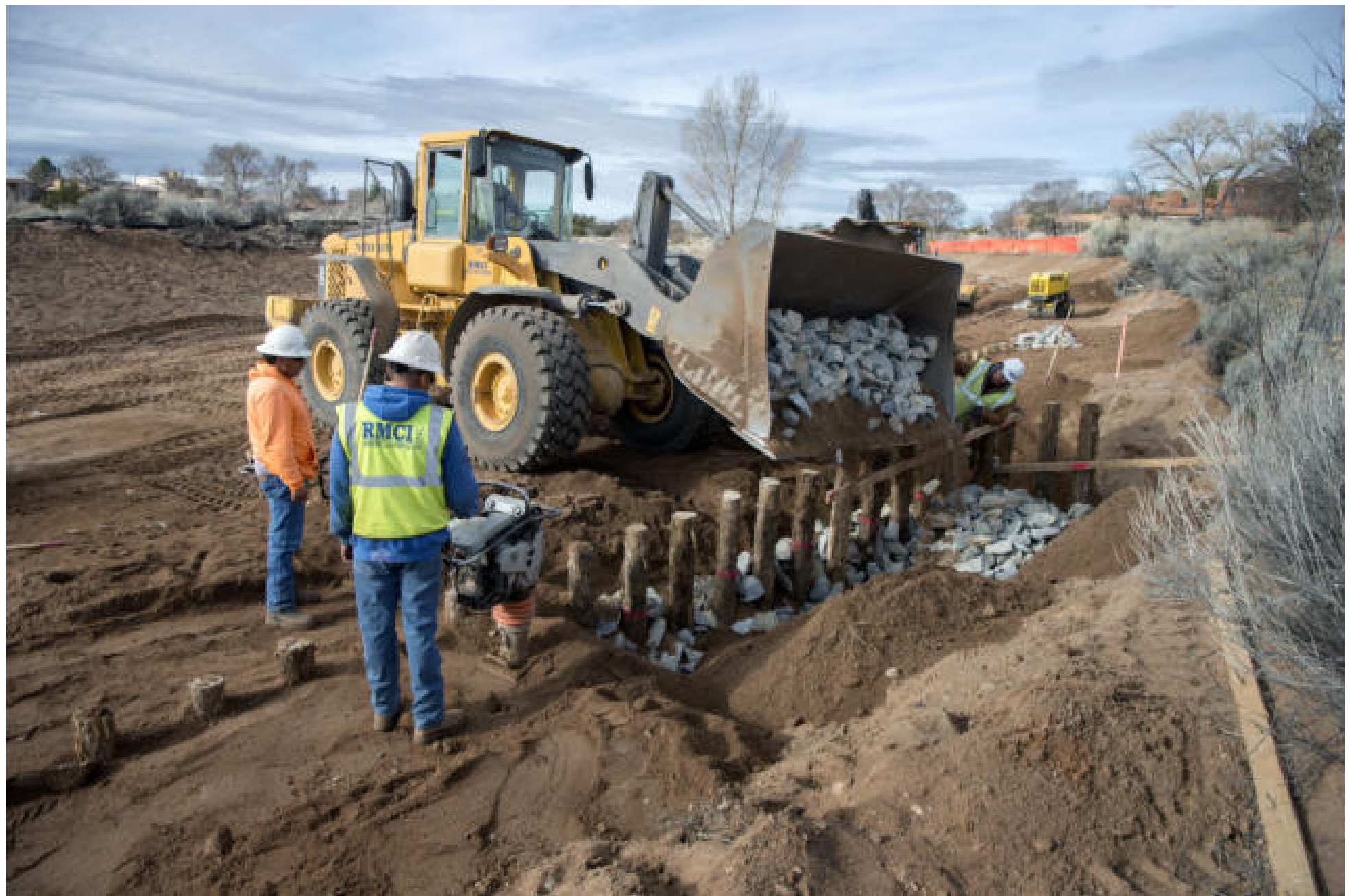
Workers with the RMCI contracting firm from Albuquerque install a post vane along the Arroyo de los Chamisos west of Yucca Street in Santa Fe, part of a project to control erosion and help develop a flood plain along the arroyo. (Eddie Moore/Journal)
